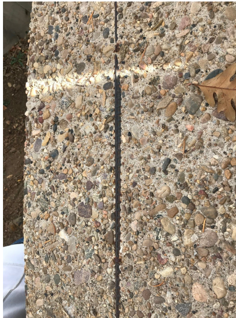
Exposed Rebar on top of the South Tank
