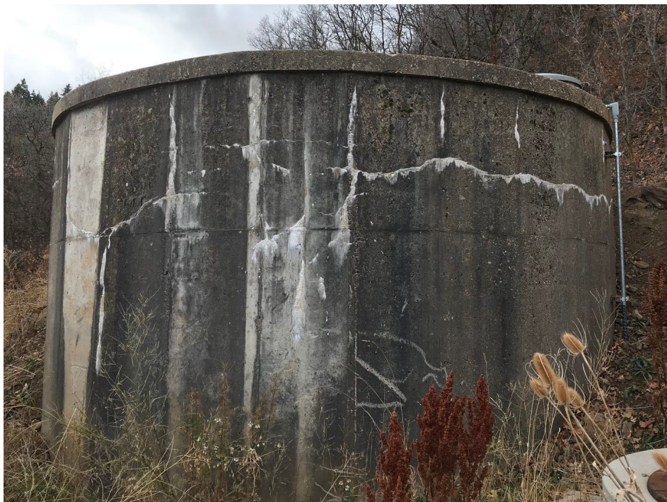
South Tank - Raw Water
