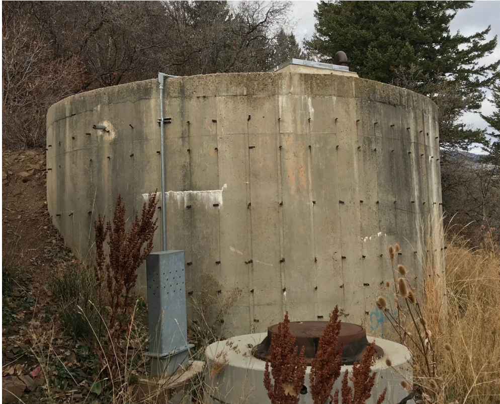
North Tank - Treated Water
