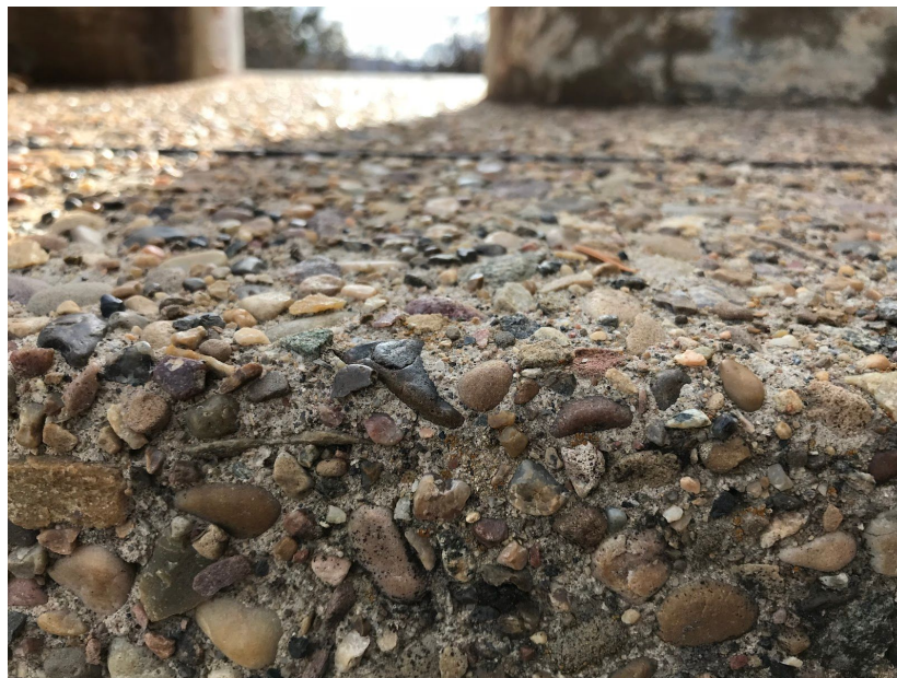
Spalling on top of the South Tank
