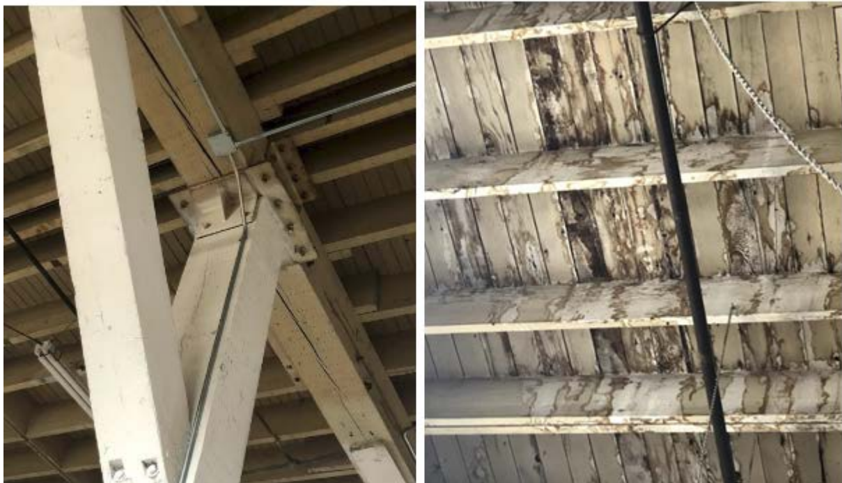
Figure 3: Split (right) and Water Damaged (left) Members
