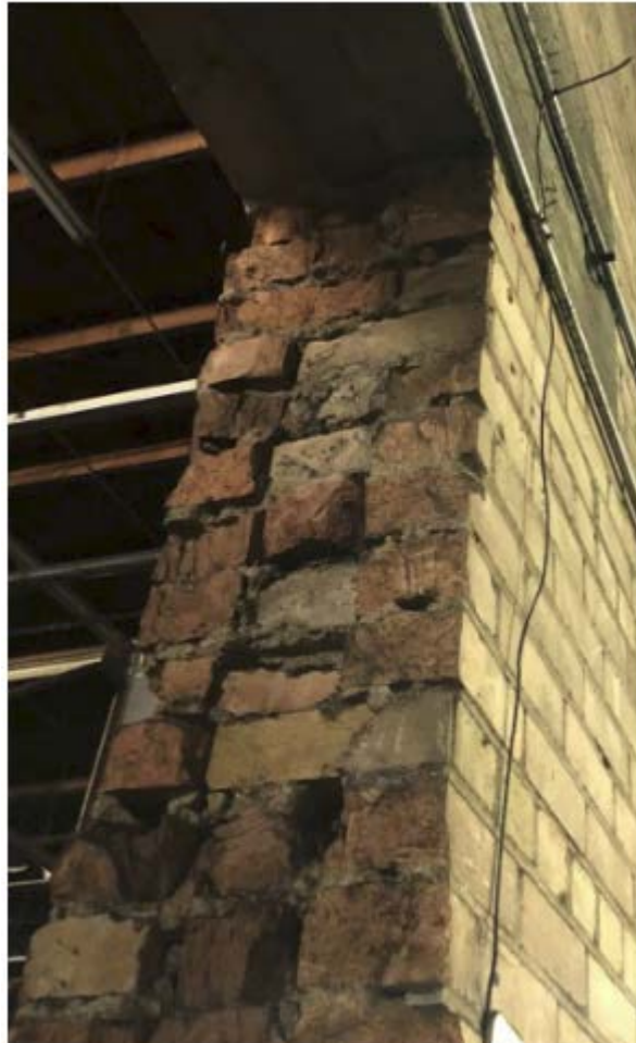
Figure 6: Masonry Wall with No Visible Reinforcement
