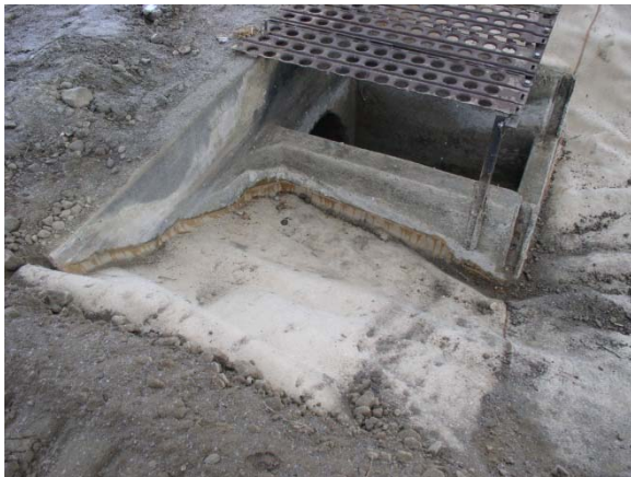
Canal 3 glued to the side of the wall
