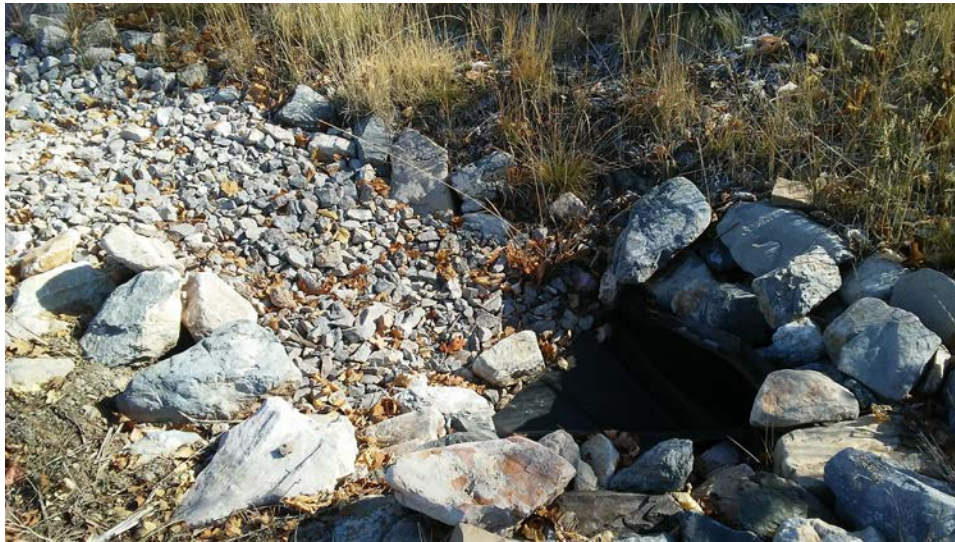
Figure 10: Existing riprap entered a mitered culvert.
