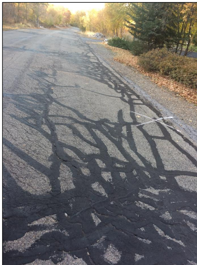
Figure 1. West Spring Drive Surface Condition.
