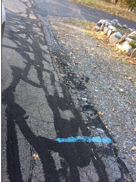
Figure 2. West Spring Drive Surface Condition
