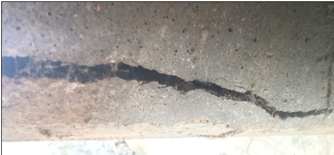
Figure 15: Large Developing Crack, January 2019
