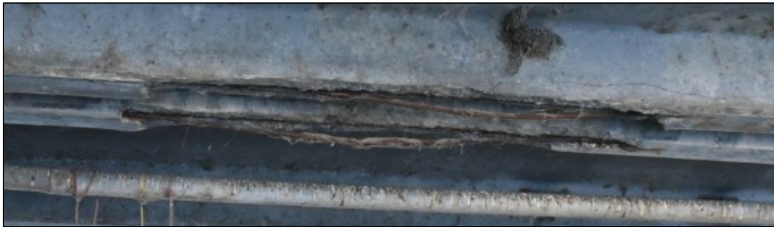
Figure 12: Corrosion on Girders 8 & 9, October 2018
