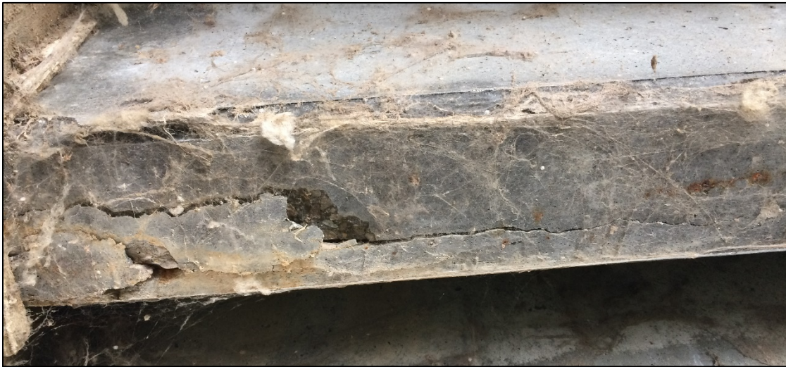
Figure 19: Other Cracking and Delamination, January 2019
