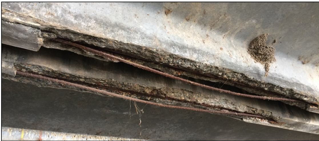
Figure 13: Corrosion on Girders 8 & 9, January 2019
