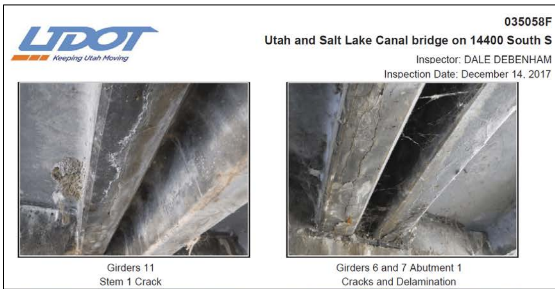
Figure 16: UDOT Inspection Report Cracking, 14 December 2017
