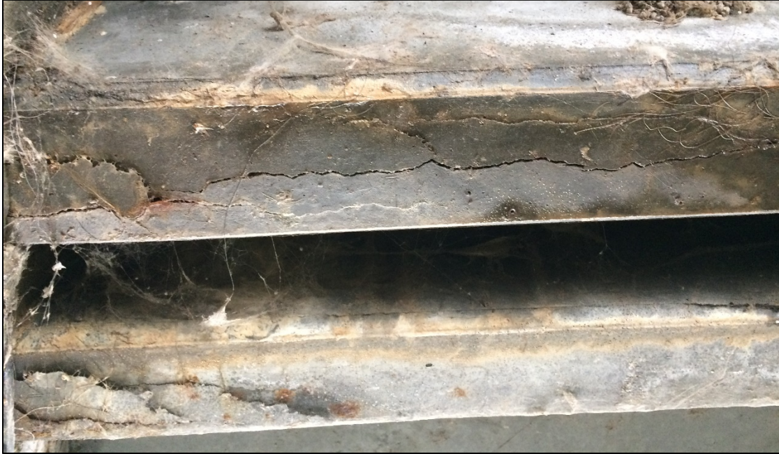
Figure 18: Girders 6 & 7 Cracking and Delamination, January 2019
