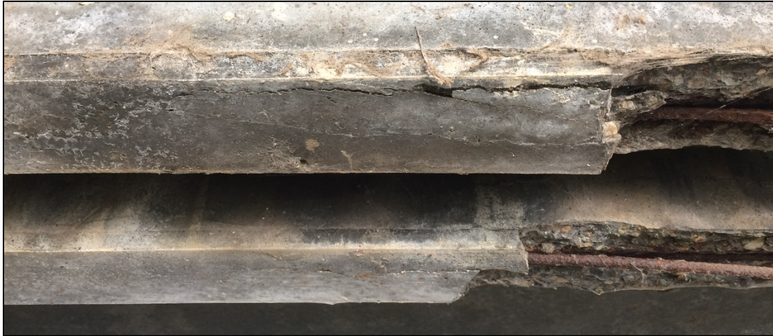
Figure 14: Close-Up of Corrosion, January 2019
