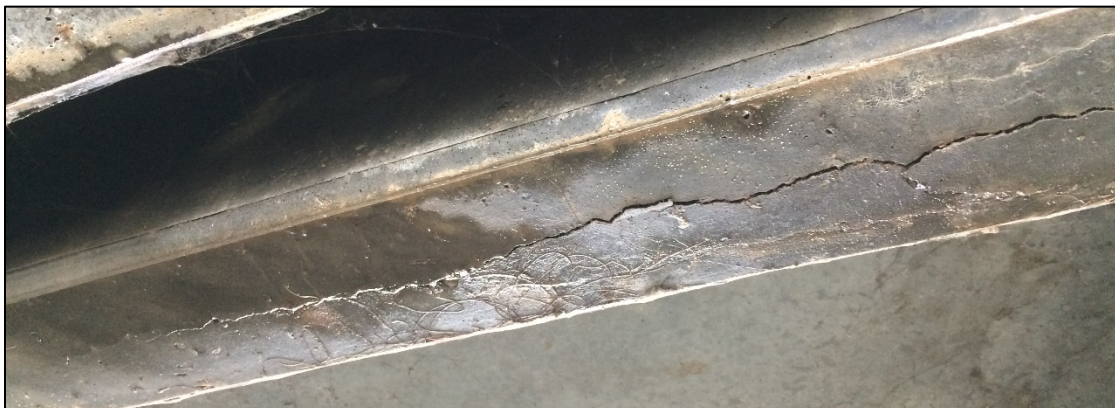
Figure 17: Girder 6 Cracking Near Mid-Span, January 2019
