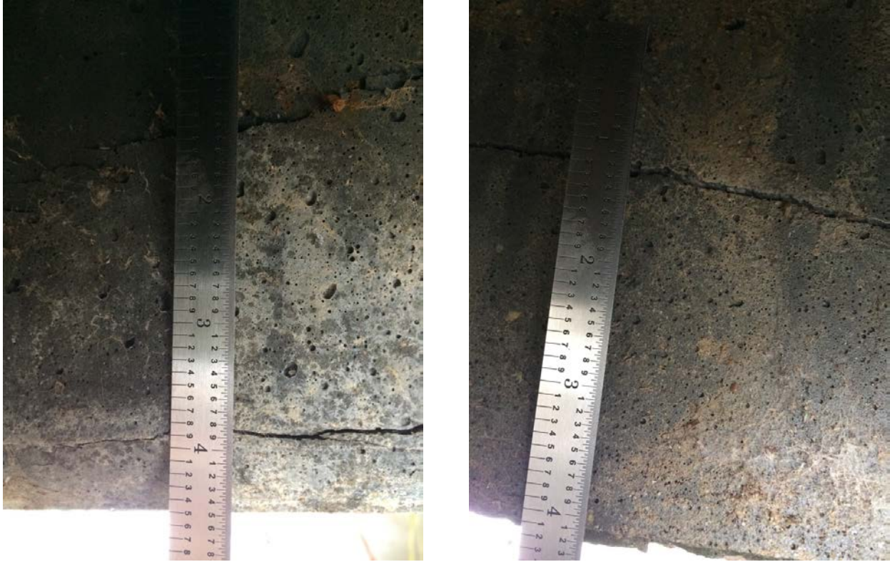
Figure 21: Primary Crack Concern, January 2019
