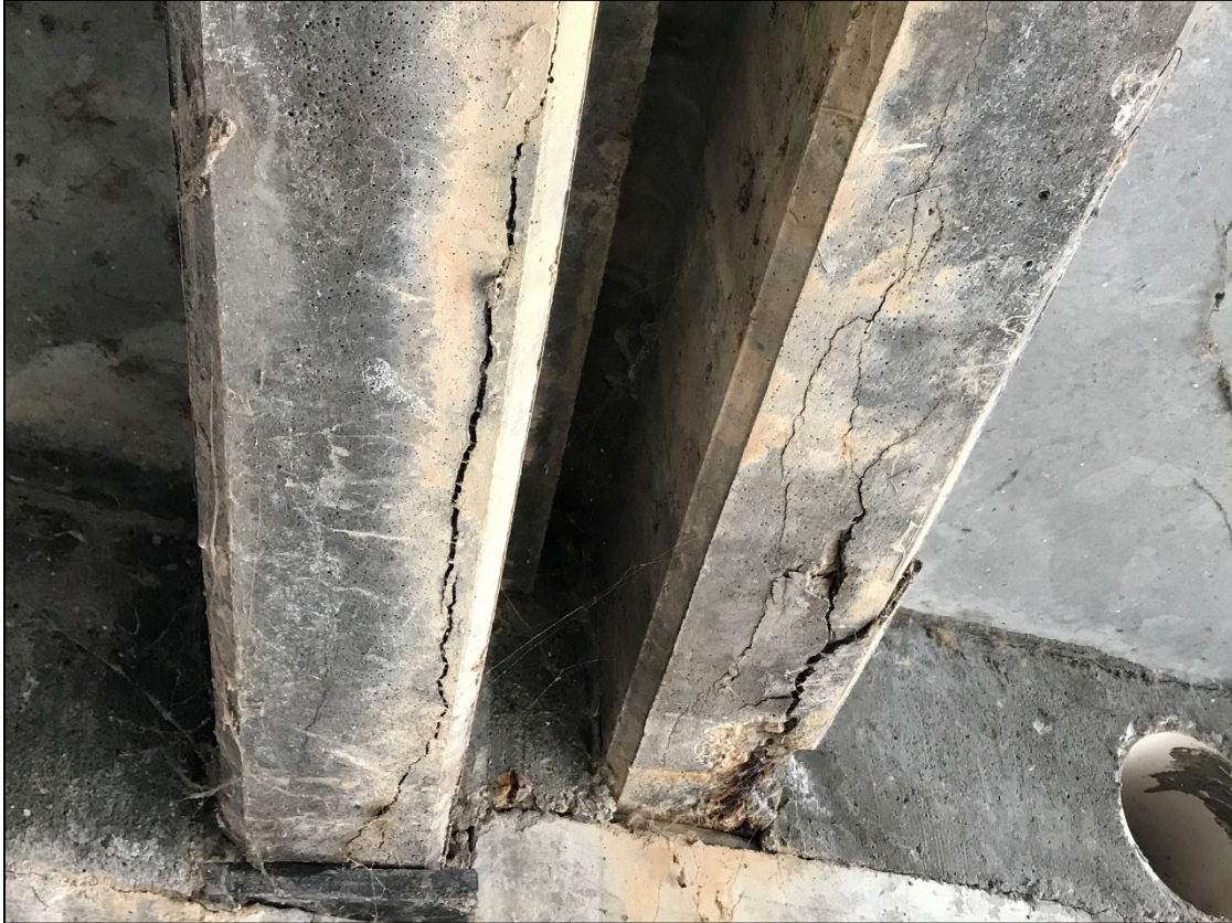
Figure 20: Girders 10 & 11 Cracking, March 2019
