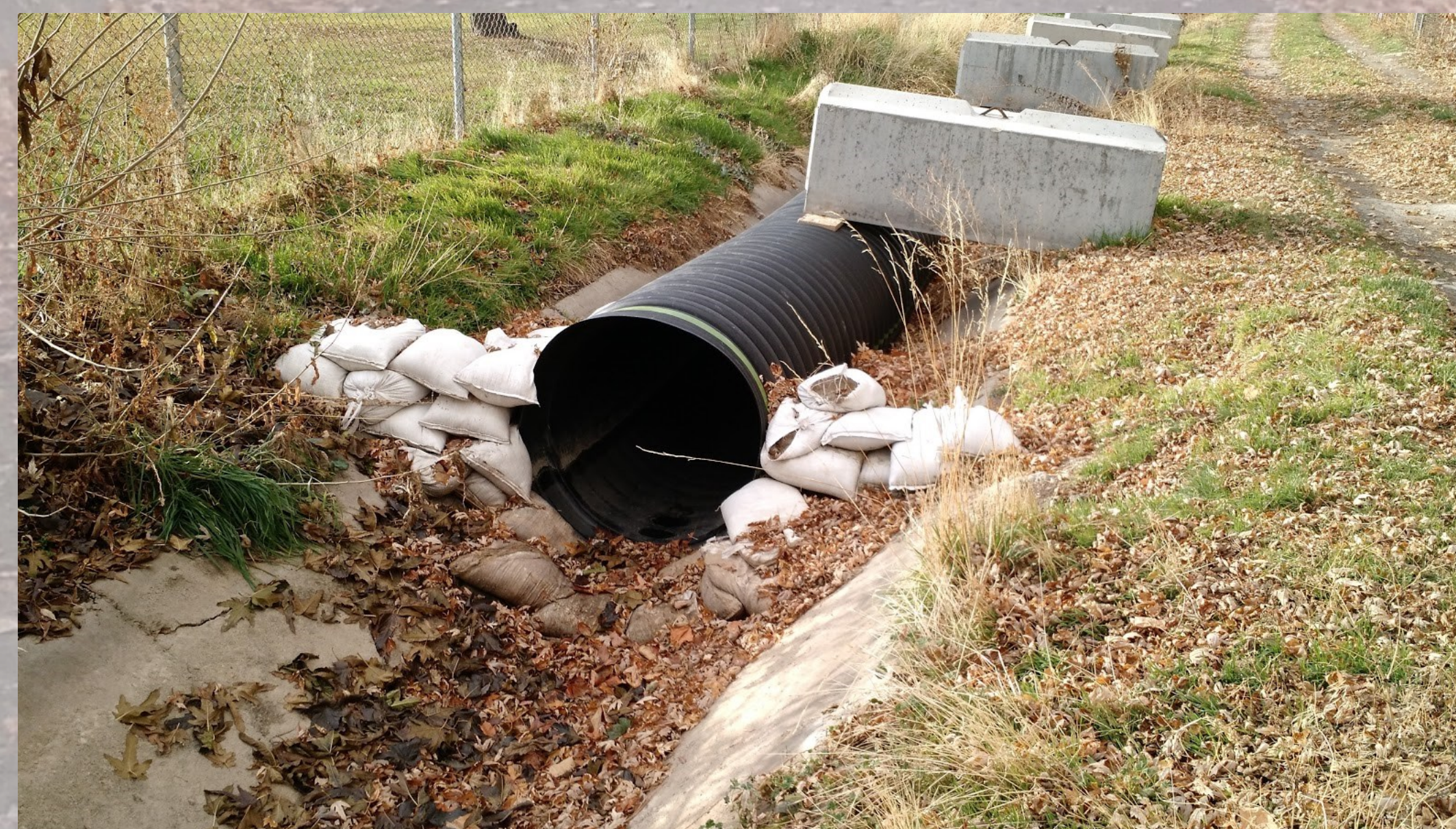
Severe canal damage in expansive clay soil with temporary fix
