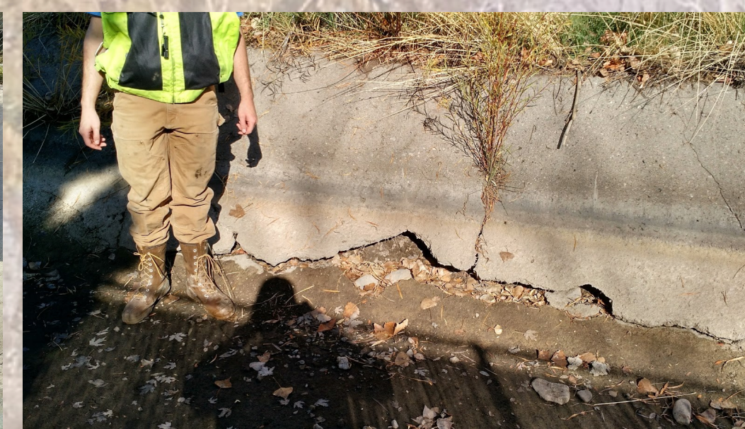
Block Faulting and erosion undermining canal lining
