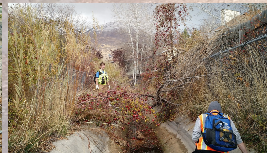
Overgrown easement encroaching on canal
