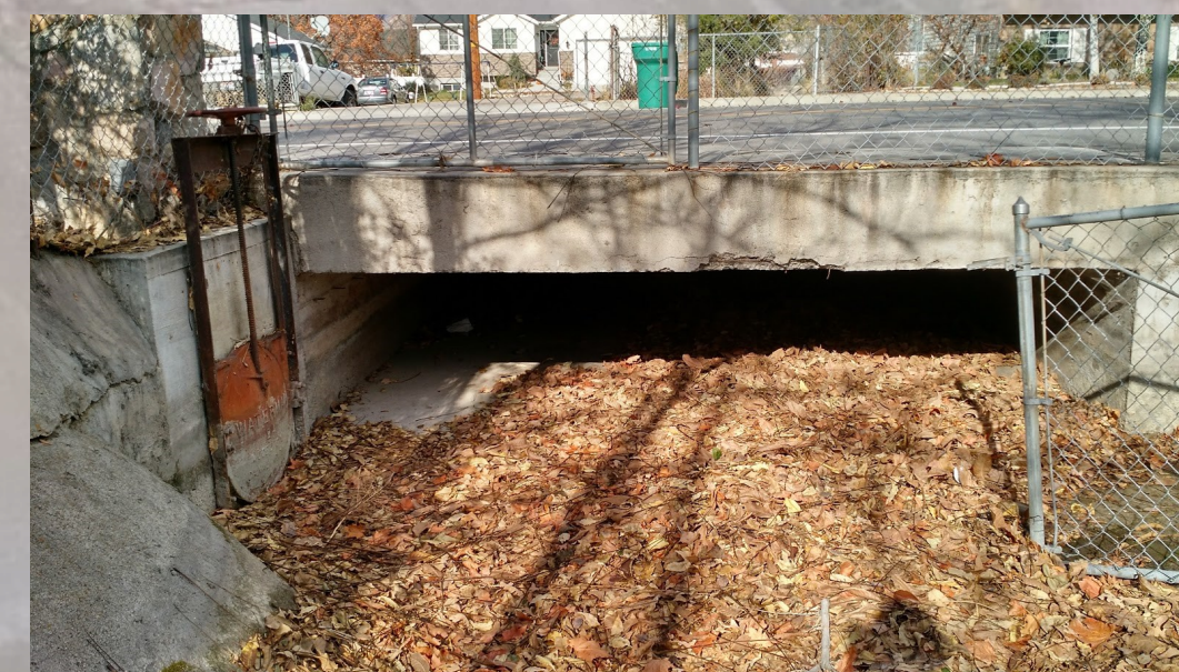
Debris clogging canal and decaying bridging structure
