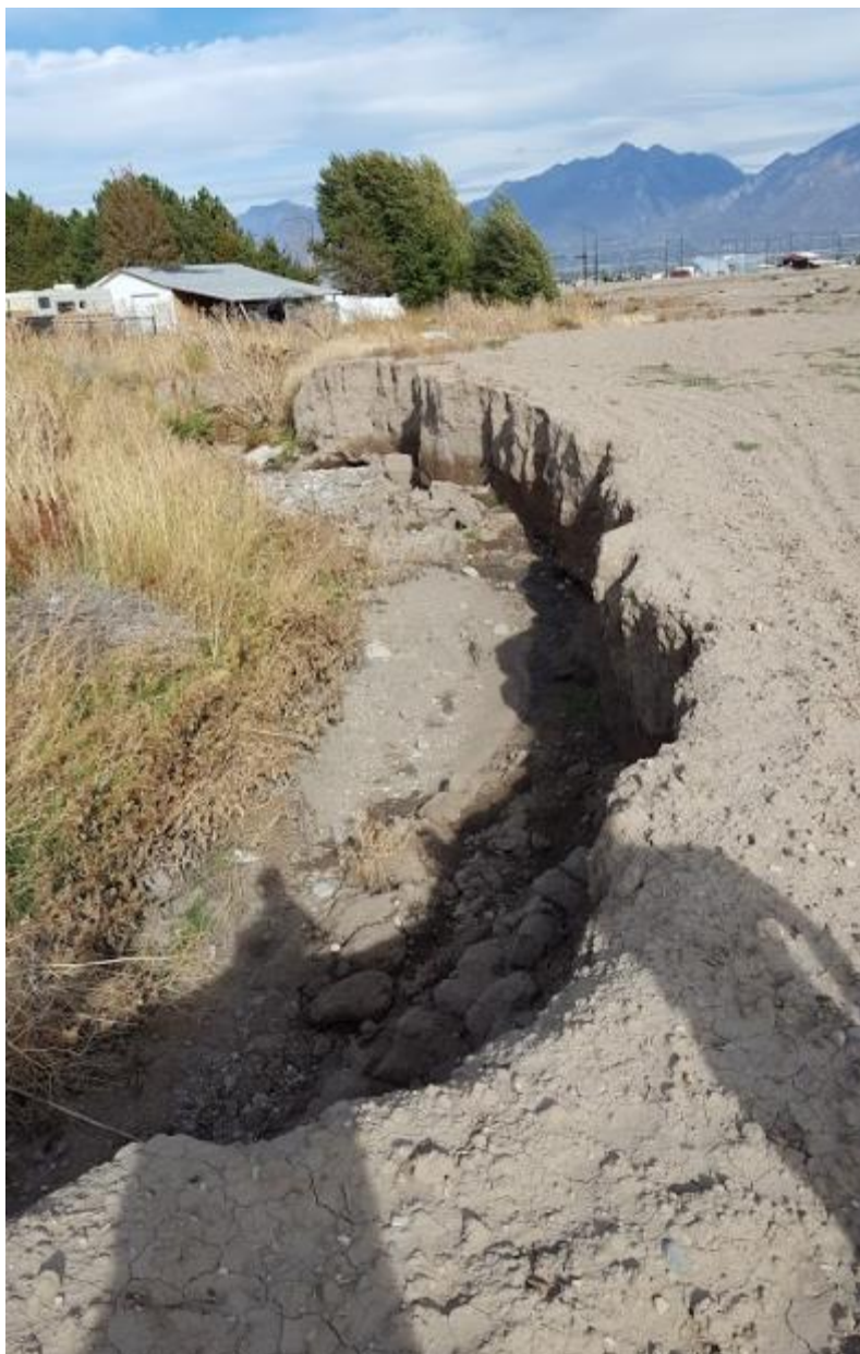
Figure 1. Image of erosion taken in October, 2016
