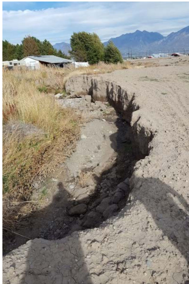
Figure 1. Image of erosion taken in October, 2016
