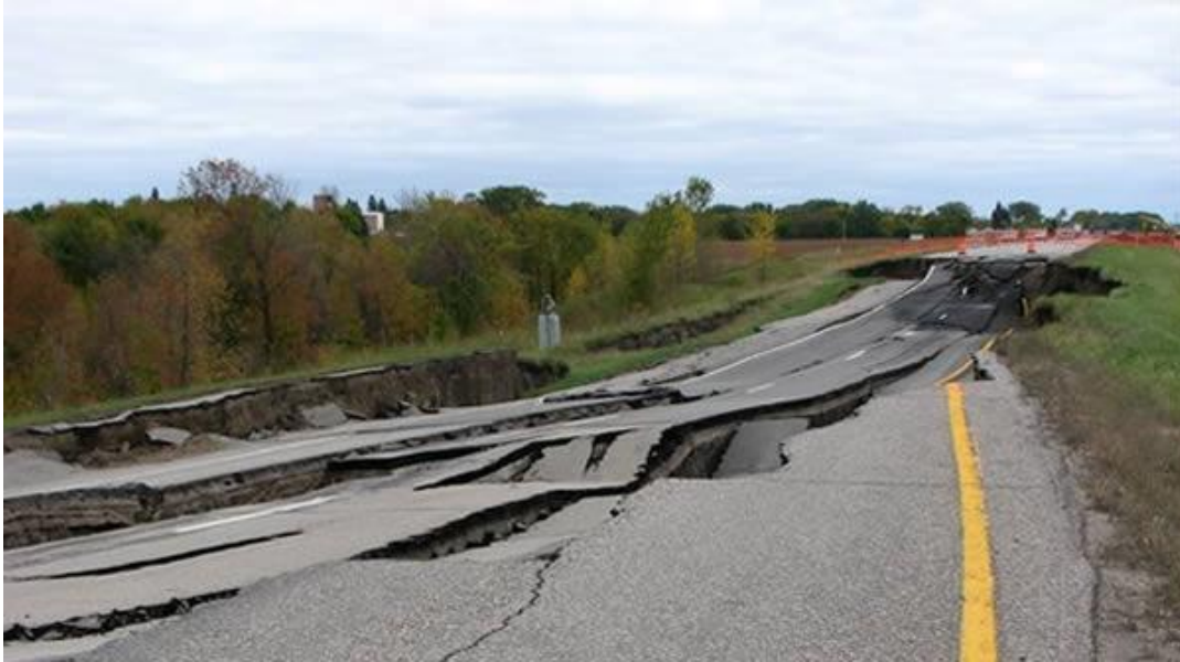
Figure 2: Damage from previous landslide (2008) on a different section of Trunk Highway 2 (Source: newsline.dot.state.mn.us ).
